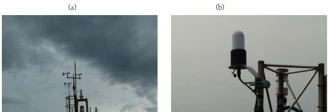
Fig. 4. The pictures of (a) wind monitor and (b) rain-gauge sensor.
